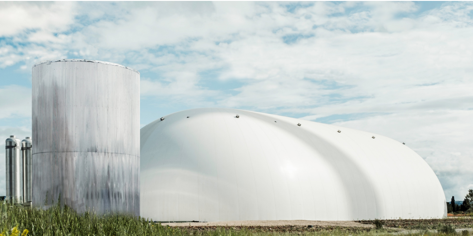
Energy Dome CO 2 battery installation in Sardinia, Italy
